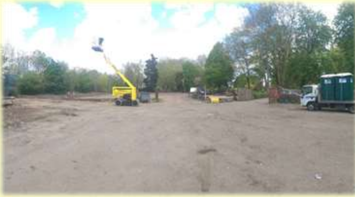
This is where our new school is going to be! Everyone has been hard at work clearing the area ready for construction.
